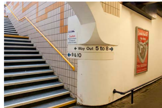
Poor alignment of information. Two different directions listed closely in the same panel.
